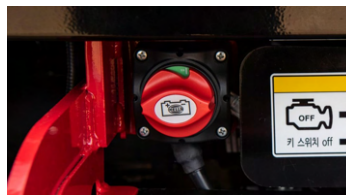
4. Battery shut-off switch
