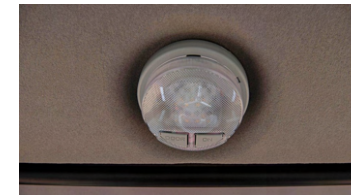
5. LED interior lighting
