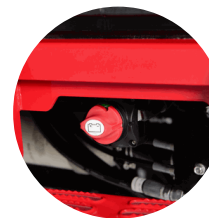
4. Battery shut-off switch
