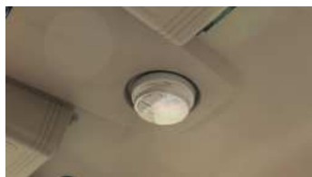
4. LED interior lighting
