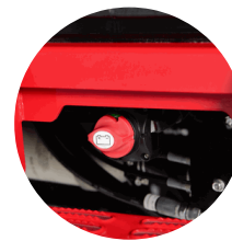
4. Battery shut-off switch
