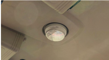
4. LED interior lighting
