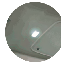
5. LED interior lighting
