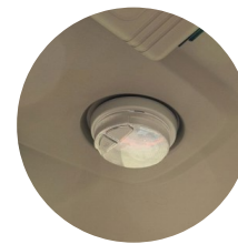
4. LED interior lighting
