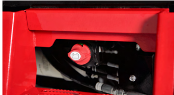
4. Battery shut-off switch
