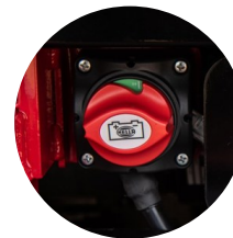
4. Battery shut-off switch
