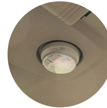
4. LED interior lighting
