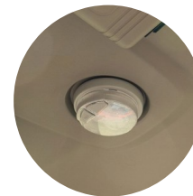
4. LED interior lighting
