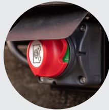
2. Battery shut-off switch
