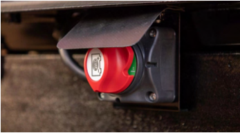
2. Battery shut-off switch
